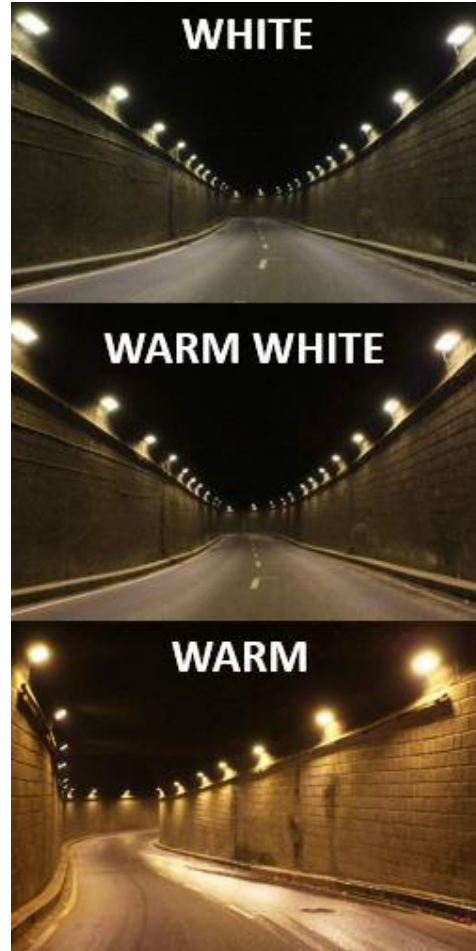
Image 2: Variations in the type of lighting in a tunnel achieved with white color tuning LEDs.
